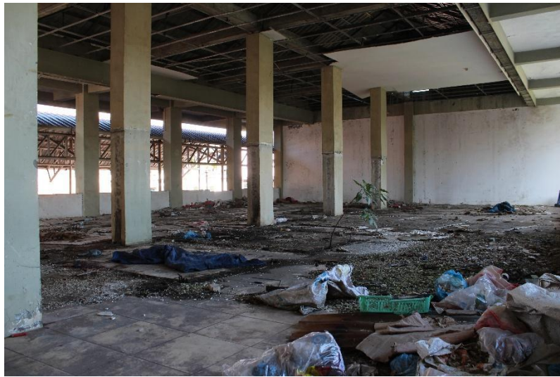
Figure 7. Pasar Kartini Abandoned Building and Waste Accumulation, July 2025
